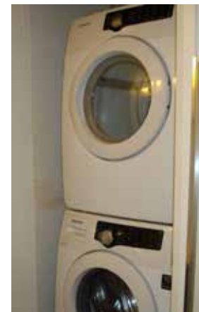
Laundry Machine shut-off valves. Typically located beside or behind laundry machine. Refer to Homeowners Manual for suggested shut off times.
