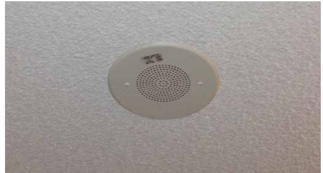
Fire Alarm Speaker – Do not disconnect
